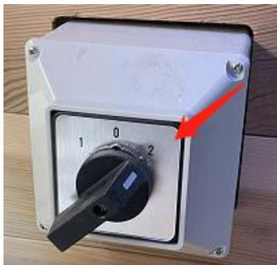
Power to Infrared heaters
